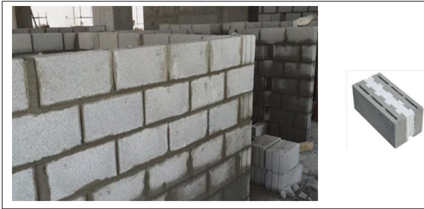
Figure 11. single wall system is made of cement bricks insulated with one slice
